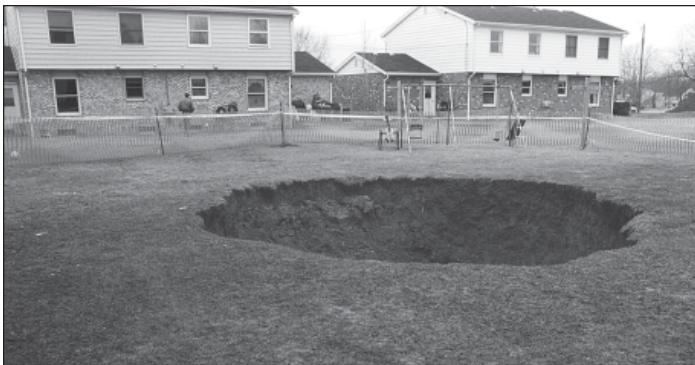
This subsidence pit behind a residence in North Canton, Stark County, was 35 feet across and 25 feet deep. Photo courtesy of Ohio Division of Mineral Resources Management.
